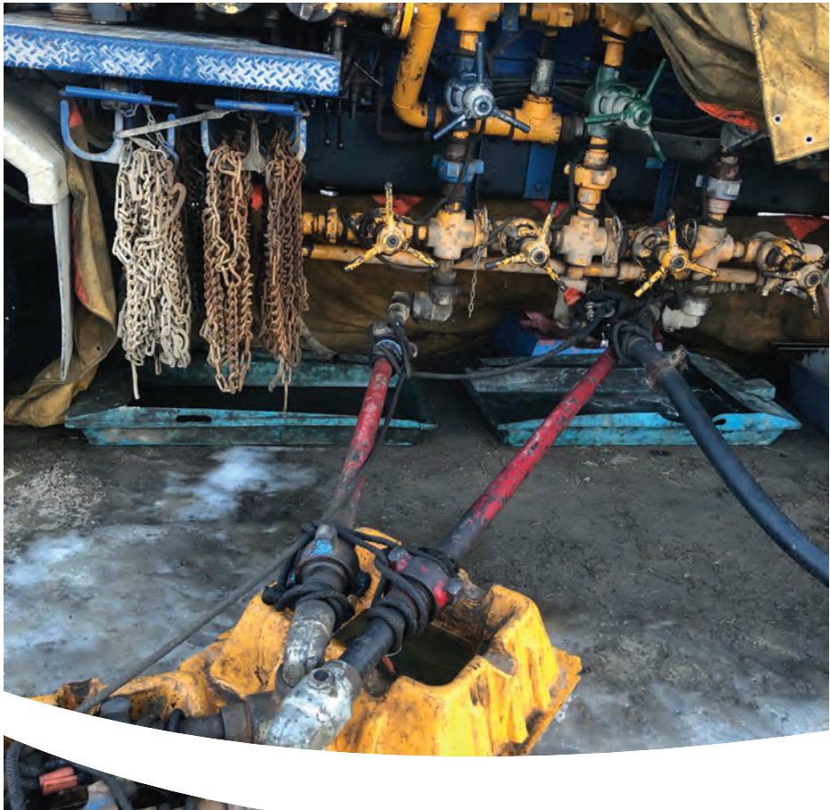
Service rig manifold, Fort Liard area, February 2022. (Credit: OROGO)
